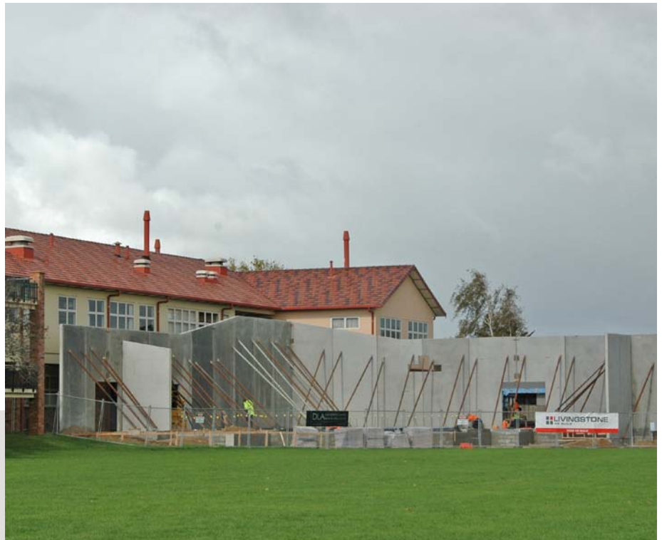
Construction is progressing well with the Gallagher Agribusiness Centre of Excellence building taking shape next to the science block.
